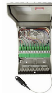
Basement RDT box
