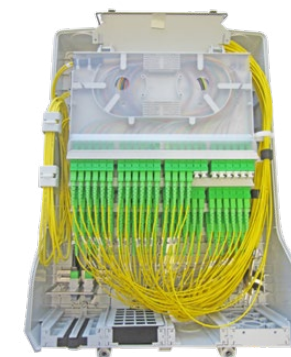
BUDI basement terminal box
