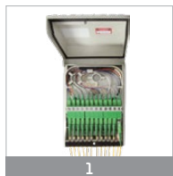
Basement RDT box
